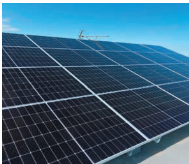
Solar panels on the roof
