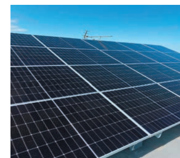
Solar panels on the roof
